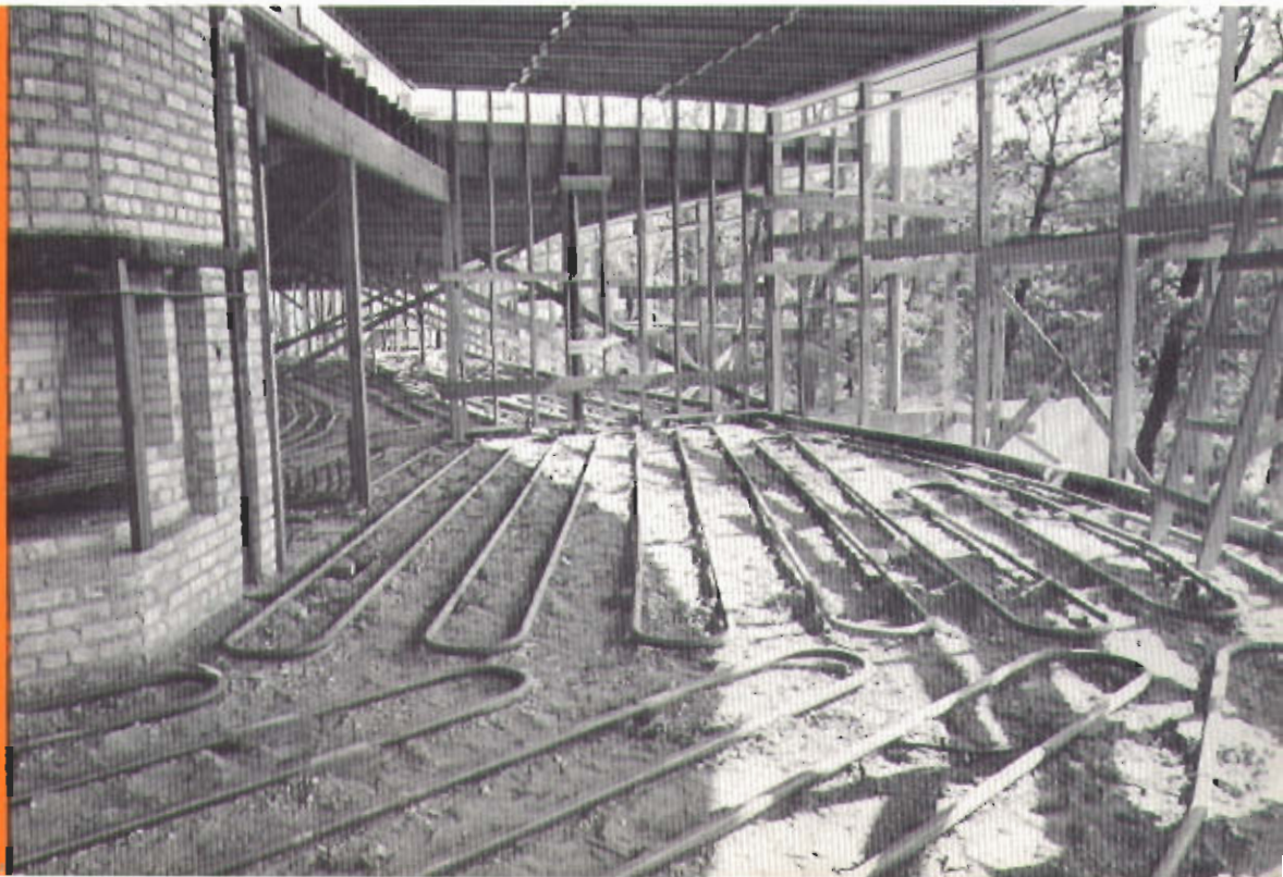
An interesting and unusual radiant heating coil arrangement, for the attractive home of J.T. Kelley, Barrington, Illinois.
