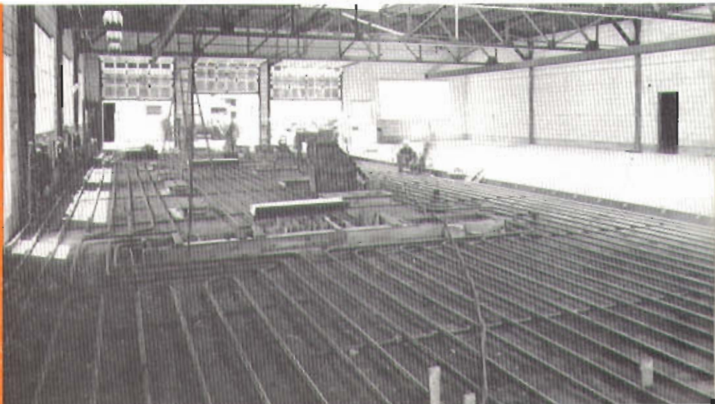
Section of Mulvihill Motor Company building in Grand Rapids, Michigan, where 6000 feet of 1\frac{1}{4} -inch National Pipe was used for the radiant heating system.
