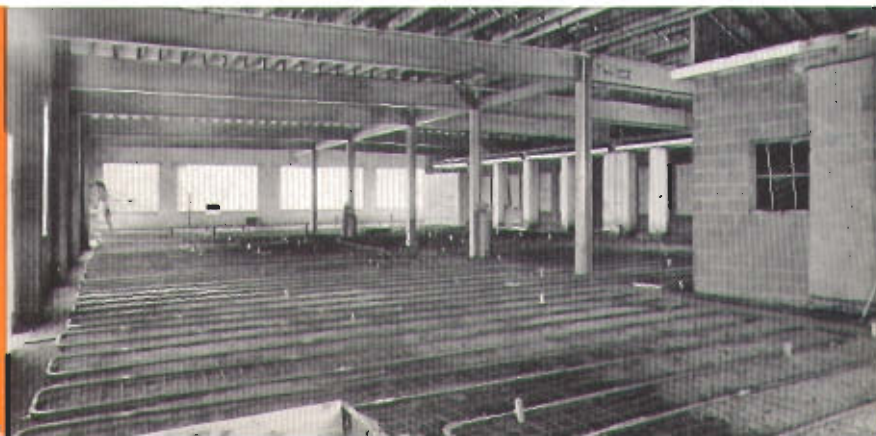
Installation of floor panel for plant of Perfection Pipe Nipple Company, Madison, Ohio. Coils are shown preparatory to laying concrete.
