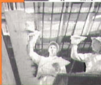
Interior view of the Jack Pahl residence, showing ceiling coils being covered with plaster.
