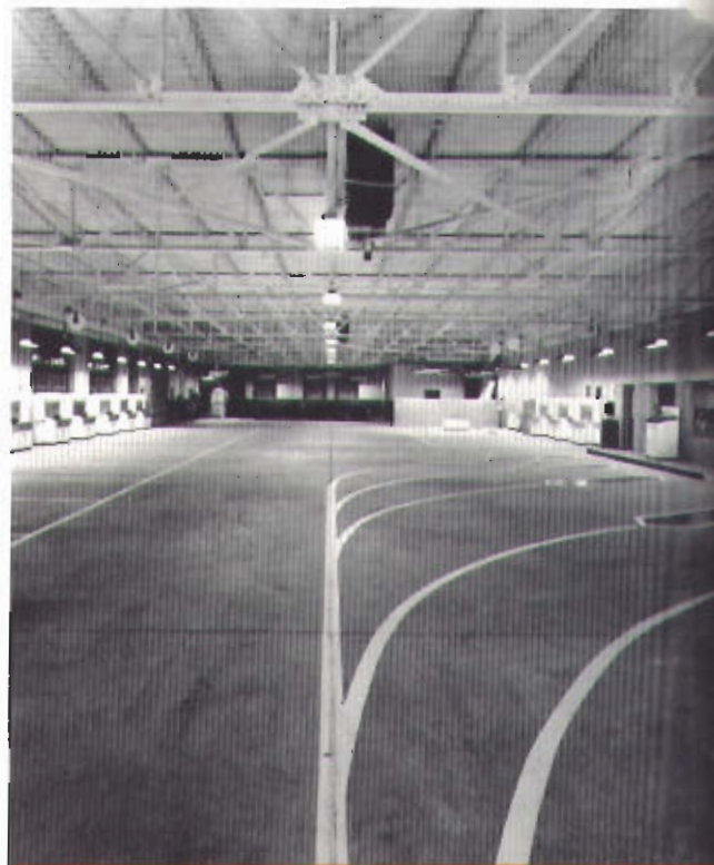
The Kuykendall Chevrolet Company garage, in Lubbock, Tex is skillfully designed with two important things in mind: efficiency for low operating cost; maximum comfort for mechanics personnel. Radiant heating is effectively used for these results.
