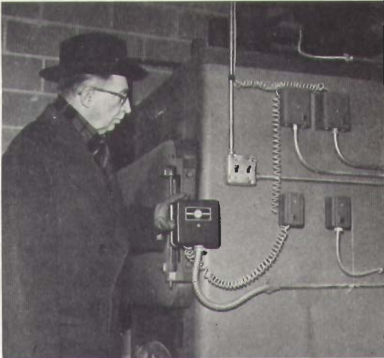
MASTER CONTROL on radiant panel heating system is checked by J. M. Wyllie, president of the transit company using the garage. Vogt installed two high-limit controls in series to keep the water temperatures below a maximum of 120F at all times, confirming his belief that plastic pipe panel jobs are all right if temperatures are controlled.
