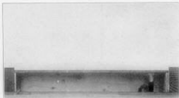
Fig. 43. Heater removed. Quarter-round on floor has not been disturbed. Opening is only \frac{3}{4} inches from floor, making possible the use of standard 8" baseboard. See Fig. 54 for details of construction of removable section of baseboard.
