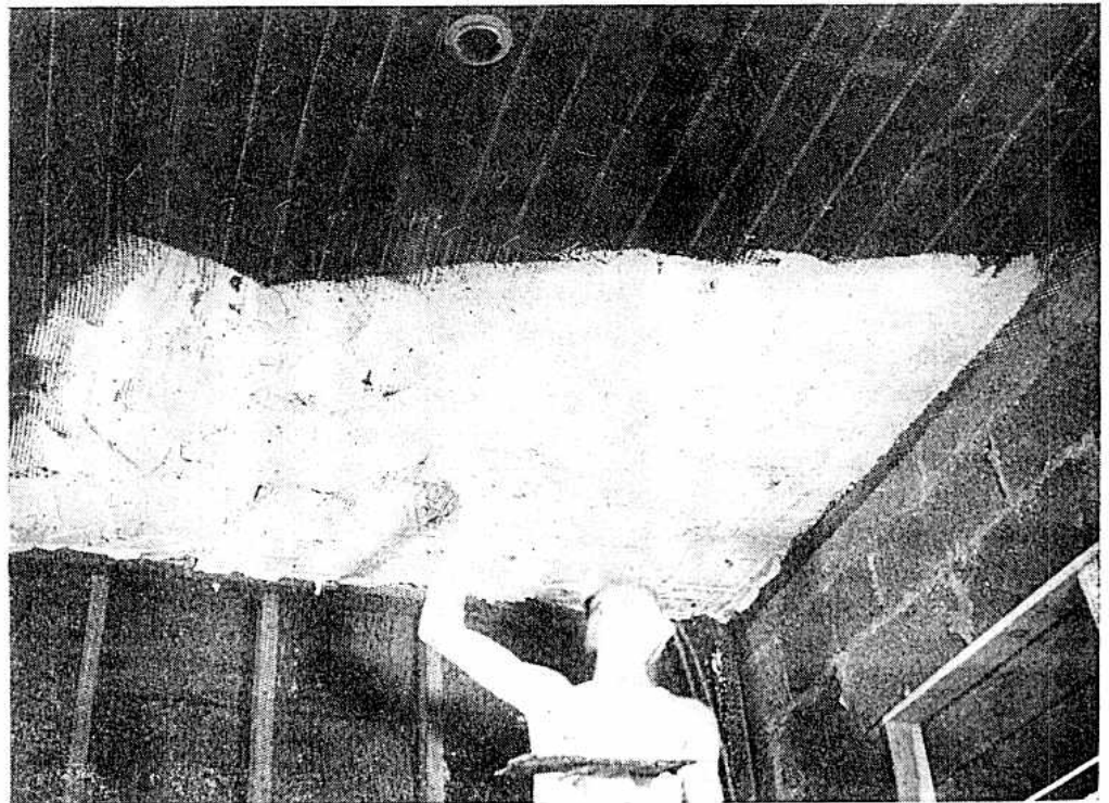
Fig. 6. Applying the scratch coat of plaster with copper tube coil on top side of metal lath.
