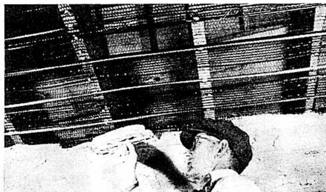
Plastering is done in the regular way just as if no radiant heating coils were installed. The plasterer thus has an unobstructed area for his work and much more uniform panel surface temperatures exist than if the copper tube were installed below the metal lath and completely embedded
