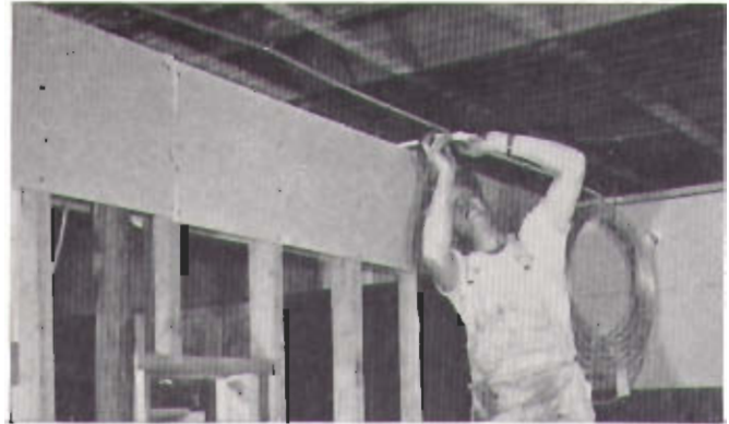
Locating the position of the first tube in the ceiling panel coil. Notice the coil of copper tube temporarily hung from the mesh with a U-hook while the measurement is being taken.
