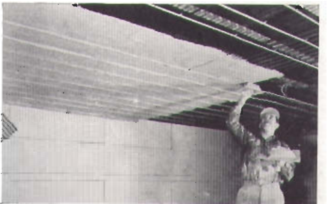
Applying the first or scratch coat of Gypsum plaster to ceiling. Other coats will follow to give final cover of 1/4" over copper tube.
