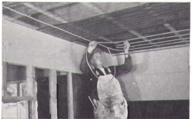
Making uniform bends by hand, to the required center-to-center distance of tubes, using a helical spring to bend the tube.
