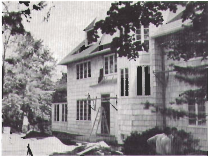
Forced hot water Radiant Heating was installed in the new addition to this house as an extension to the conventional steam heating system in use.
