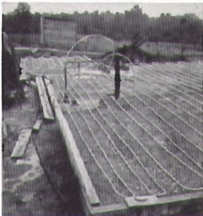
Approximately 1,200 ft. of 3/8" Type L Copper Tube was built into panel coils for this house.
