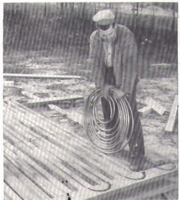
A wooden form, or mold, is quickly constructed, in sections easily moved from job to job. The workman, with a section of coiled soft copper tube starts the simple operation.
