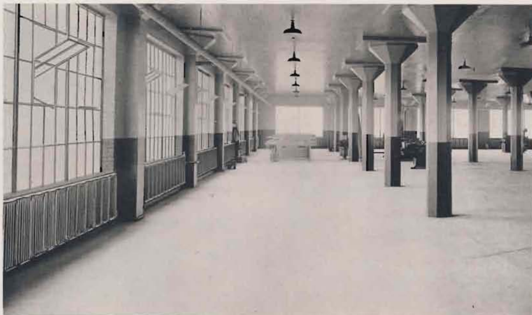
There are 60,000 feet of AMERICAN PEERLESS Wall Radiators in the plant of Central Supply Co., Saginaw, Mich.
