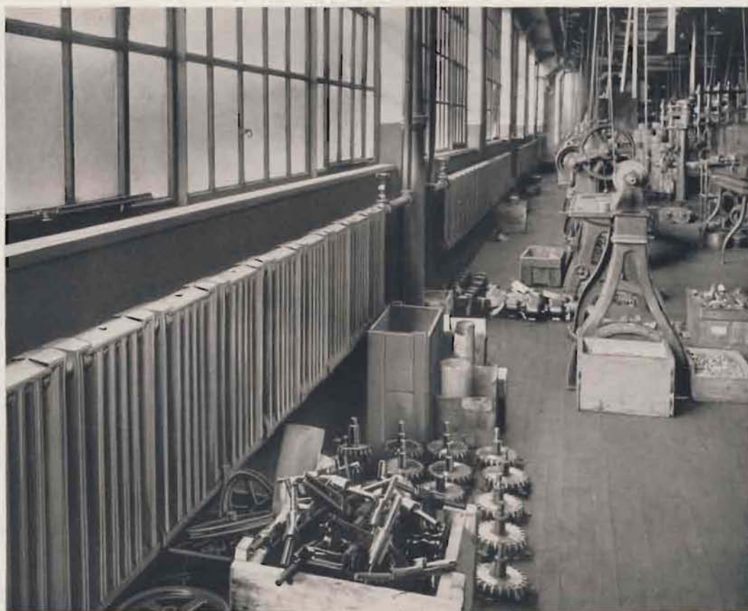
AMERICAN PEERLESS Wall Radiators installed in the plant of the Diehl Manufacturing Co., at Elizabeth, N. J. This installation is exceedingly simple and is typical of the arrangement of wall radiators in numerous factory buildings.
