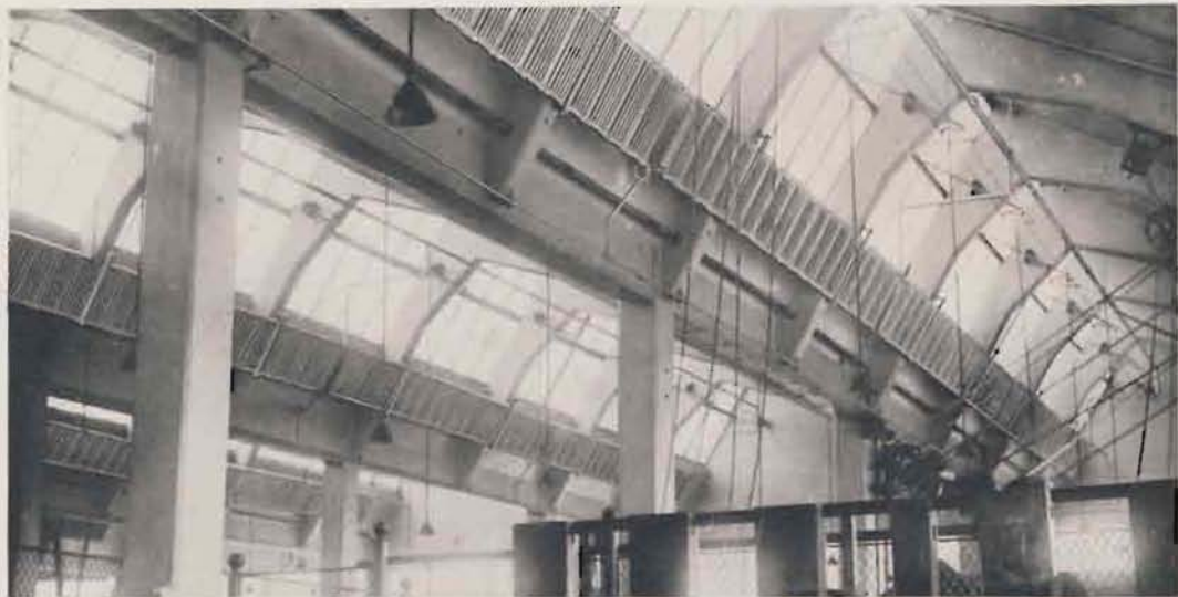
Interior of factory of Philadelphia Textile Machinery Company at Philadelphia. Note the effective placing of AMERICAN PEERLESS Wall Radiators in skylights.
