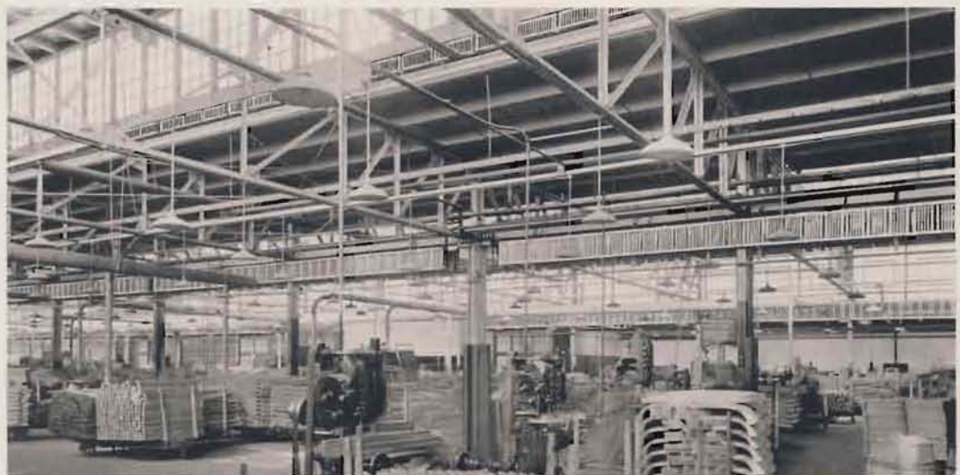
160,000 square feet of AMERICAN PEERLESS Wall Radiators used in plant of Fisher Body Corporation, Detroit, Mich.
