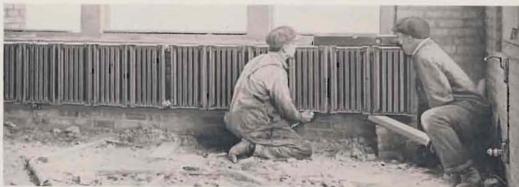
Fig. D. Using short piece of scantling as lever to level up AMERICAN PEERLESS Wall Radiators. Fitter at left with wrench tightening bolt-head of adjustable spool to level.
