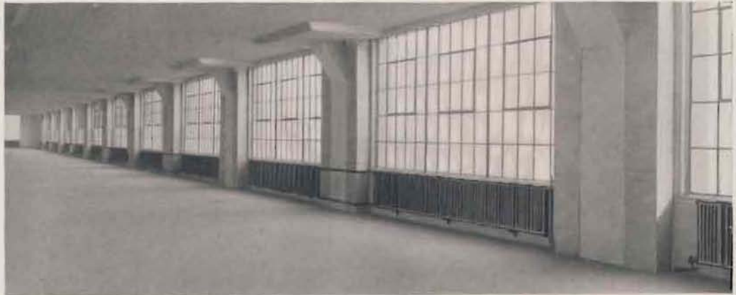
A portion of one floor in factory of Excelsior Motor Mfg. & Supply Co., Chicago. 36,000 square feet of AMERICAN PEERLESS Wall Radiators supported on ARCO Adjustable Brackets are installed in this modern reinforced concrete building. Note how these radiators conform to the design of this fire-proof construction.
