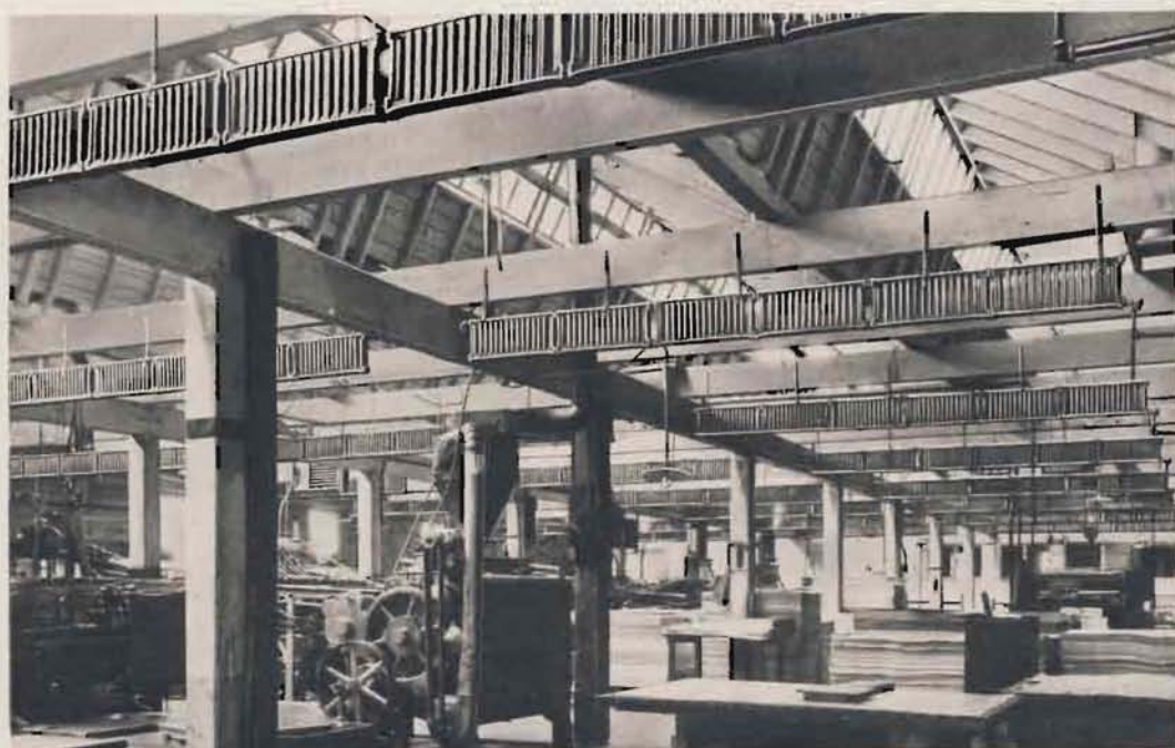
Installation of AMERICAN PEERLESS Wall Radiators in plant of Muirson Label Corporation at San Jose, Calif., showing a very satisfactory method of counteracting the cooling effect of a saw-tooth roof, insuring even heat over a large floor area.
