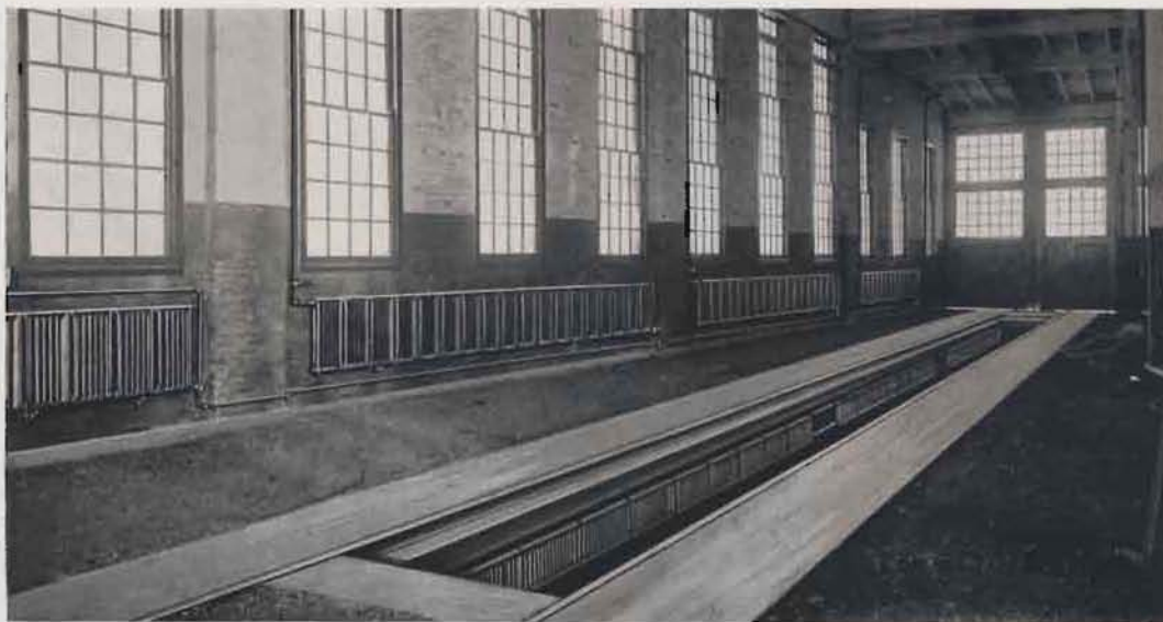
Illinois Central R. R. Roundhouse. Note the use of AMERICAN PEERLESS Wall Radiators, with ARCO Adjustable Brackets under windows and in the pits for cleaning cars of ice and snow. See details of the space-saving feature on page 11.
