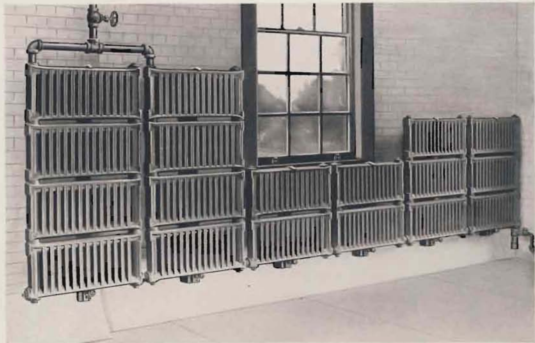
View of an effective and compact installation of AMERICAN PEERLESS Wall Radiators on ARCO Adjustable Brackets around a window, in factory of Merk & Co., Rahway, N. J. Note how the radiators are held up off the floor and close to the wall. Such distribution of radiation by means of pipe coil would hardly be feasible.
