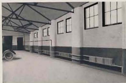
Garage at Nottingham, England. Heated with AMERICAN PEERLESS Wall Radiators, and showing a neat way of connecting up flow and return piping around pilasters.
