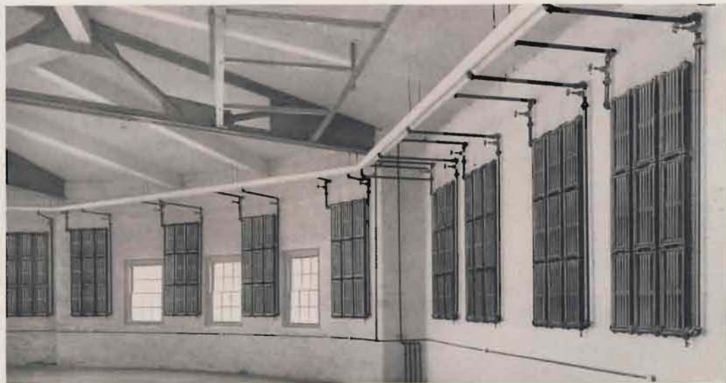
Garage of the National Electric Lamp Company, at Cleveland, Ohio, heated with AMERICAN PEERLESS Wall Radiators, arranged in separate units for heat control. Forced circulation of hot water with overhead supply and return.
