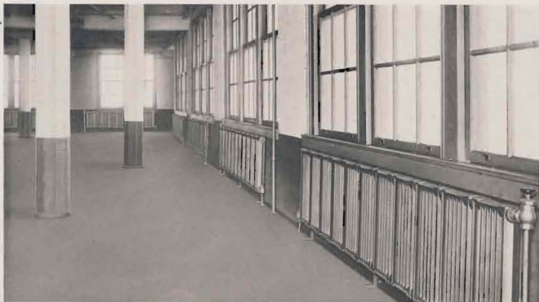
This is a typical floor and heating arrangement of AMERICAN PEERLESS Wall Radiators in the building of the Coca-Cola Company, at Baltimore. Over 60,000 square feet used.
