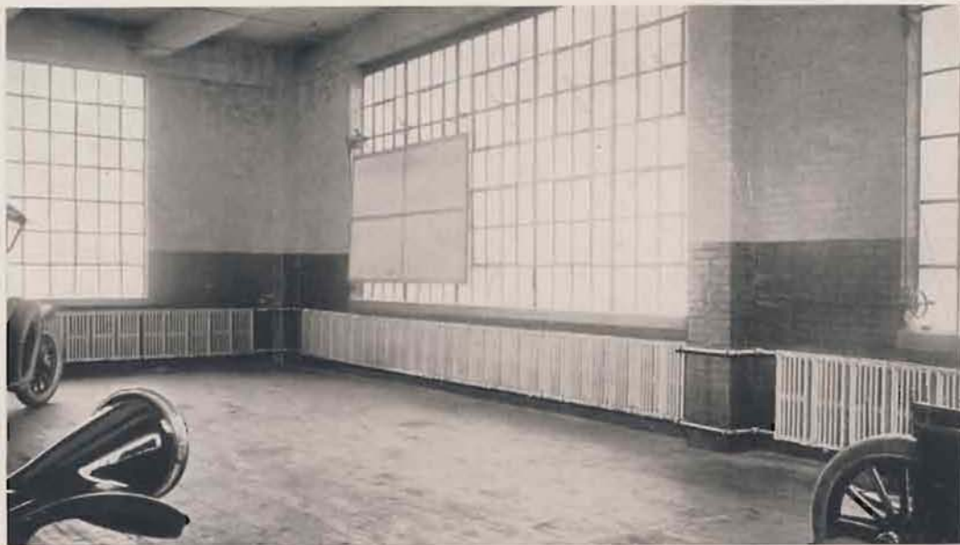
AMERICAN PEERLESS Wall Radiators in the new building of the Pierce-Arrow Company, Long Island City. Forced Hot Water circulation. The radiators fit snugly against the walls, saving space and not obstructing the light.
