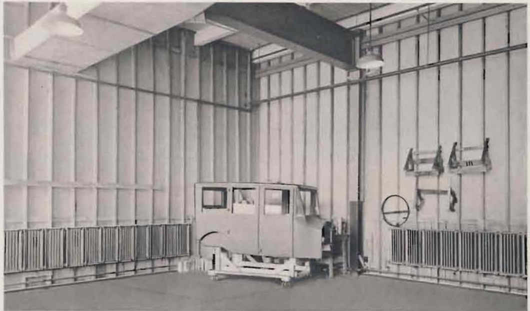
AMERICAN PEERLESS Wall Radiators in Finishing Room of Liberty Motor Car Co., Detroit, Mich.
