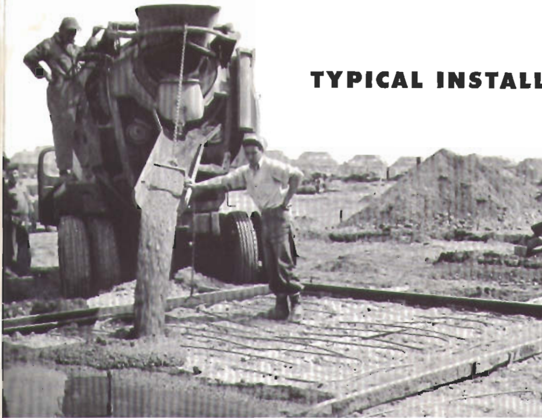
Pouring concrete over the copper tube floor coils at a large housing development on Long Island.
