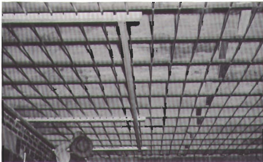
FIG. 8. WOOD FRAME FOR HANDLING SINGLES RADIANT HEATING COILS USING COPPER WATER TUBES
