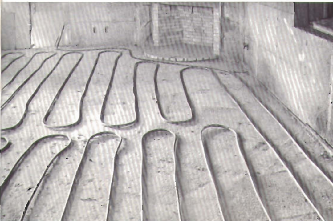
The rumpus room floor panel shown with \frac{3}{8} " soft copper tube on 14-inch centers, is typical of the other eleven panels used to heat the ground floor in a large, modern, midwestern residence. Laid on a 4" concrete slab, the coils are embedded in 3" of concrete with a terrazzo surface finish.
