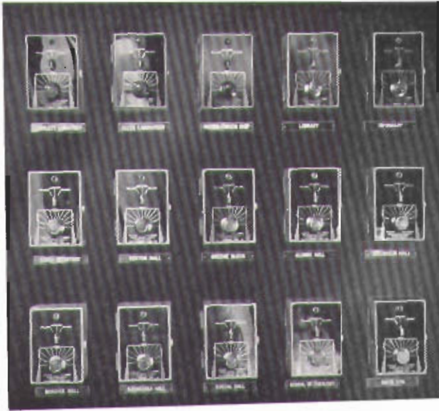
Fig. 10. Fifteen buildings at Alfred University, Alfred, N. Y., are controlled from this panel which holds 15 Webster Variators of the Type E-4 Moderator System.
