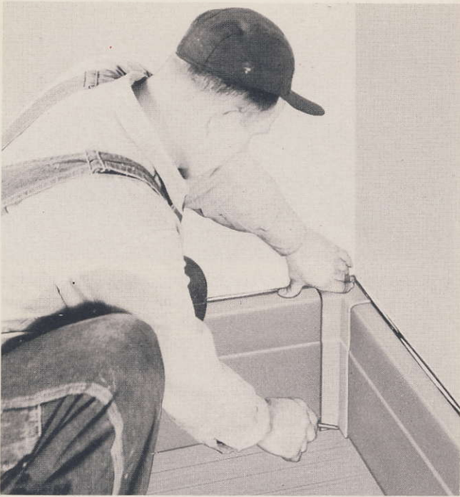
Fig. 9: Corner cover plate is held in place by wood screw in floor.
